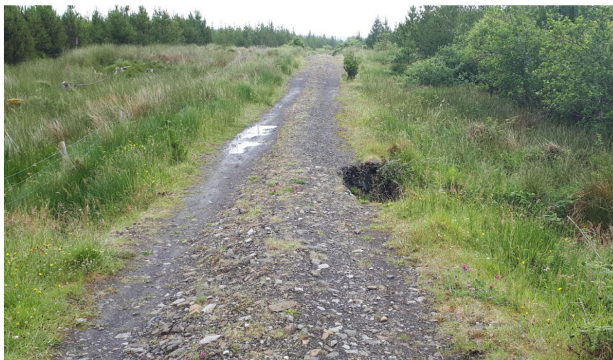
Photo 1: Road slump at culvert location (Source: FT, 2022)
